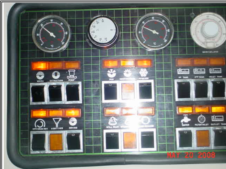
Photo of refrigerated condenser temperature gauges at start of dry cleaning cycle. left gauge indicates 38 degrees C; right gauge indicates 32 degrees C.
