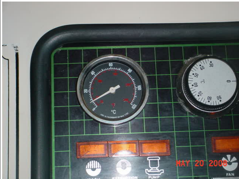
Left refrigerated condenser temperature gauge indicating 7 degrees C at end of dry cleaning/cool down cycle.
