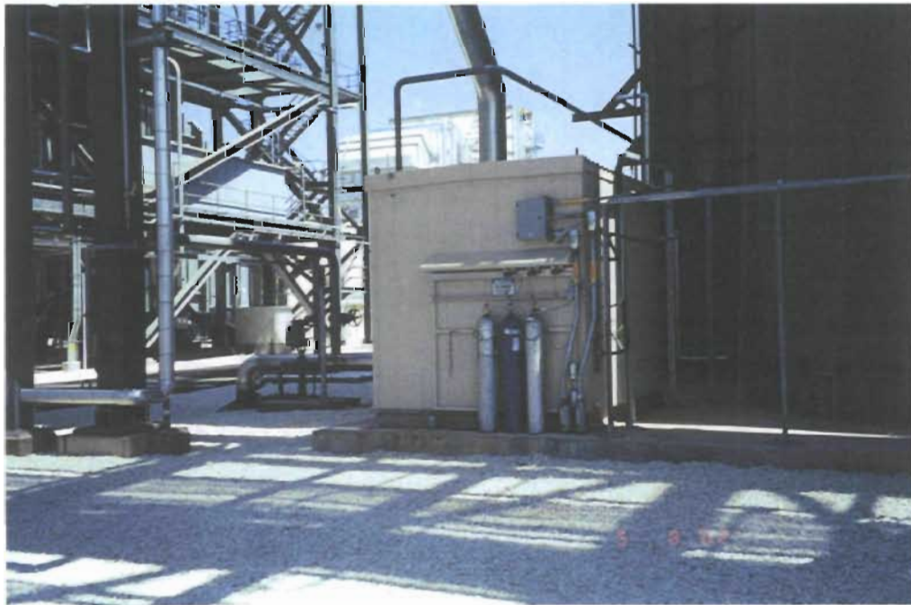
Unit 5A CEM Shelter
