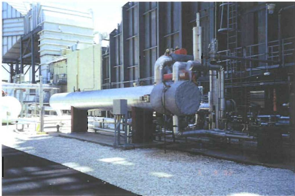
Unit 5A Steam Gas Heater
