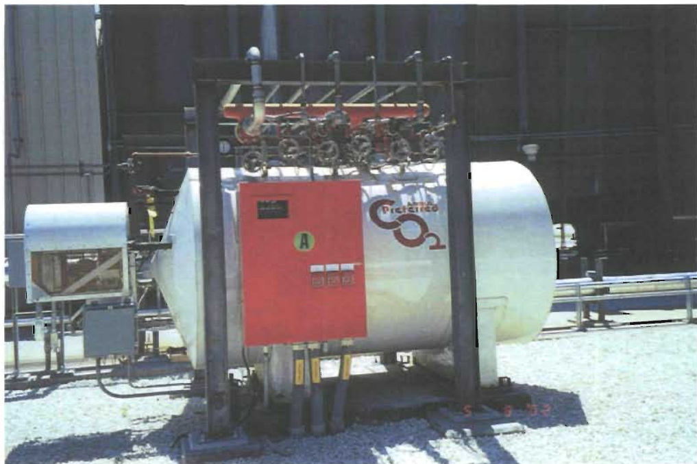
Unit 5A Fire Protection System
