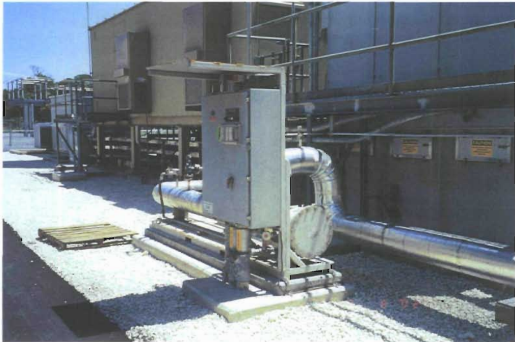
Unit 5A Electric Gas Heater (used for startup)
