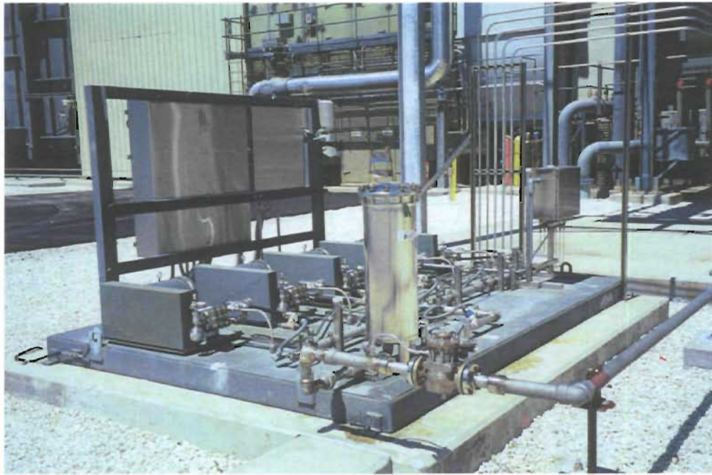
Unit 5A Inlet Fogger Skid
