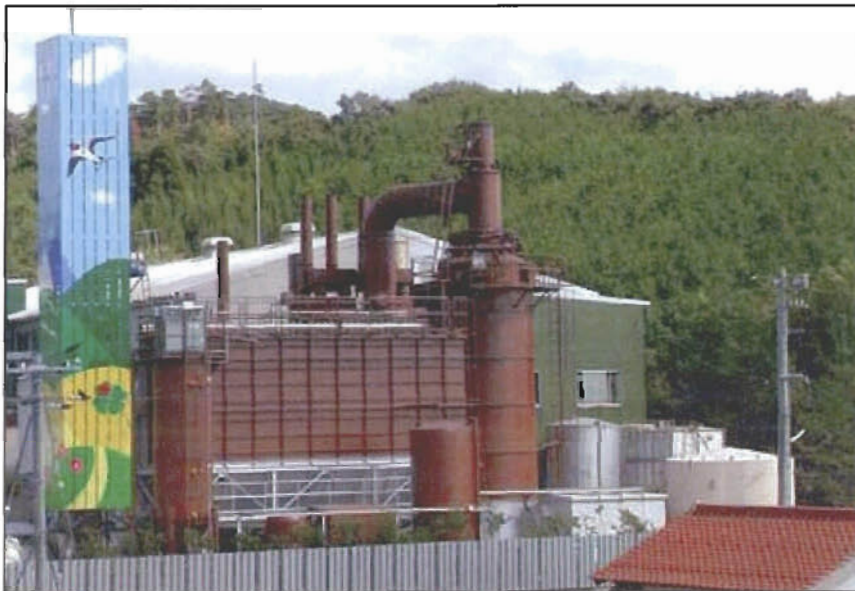
FIGURE 3. This is a general view of the filter plant and direct cooling chamber at Honshu I. The ceramic filter plant can be seen center left in the plant. To the right of the filter plant is the direct cooling chamber and to the left the exhaust stack
