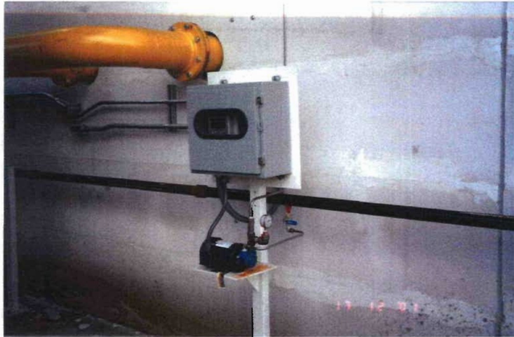
Photo 1. Front View - Selective Catalytic Reduction Control System
