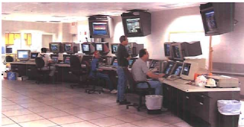
Figure 1-27 DCS Control Console
