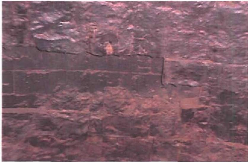
Figure 1-10 Missing Gasifier Hot Face Refractory Brick The Back-Up Brick Liner Is Still Intact
