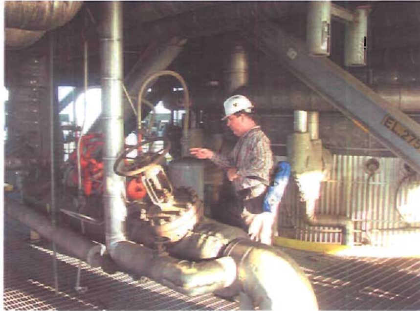
Figure 1-12 Sootblower Valve Station and Headers A Water Cooled Sootblower Nozzle Can Be Seen Behind the Escape Pack
