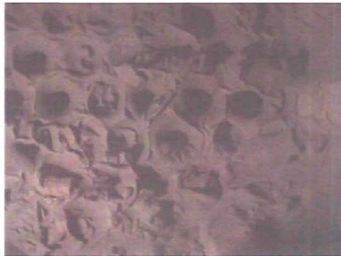
Figure 1-9 Plugged CSC Inlet Tubesheet
