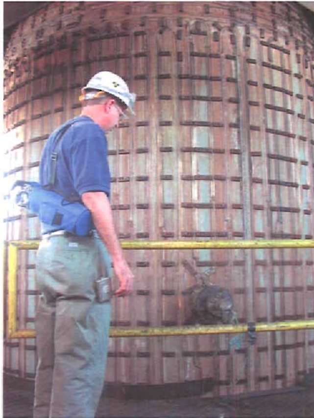
Figure 1-7 Gasifier Shell Temperature Sensing System
