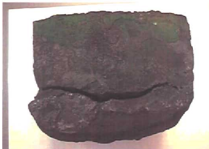
Figure 1-11 Gasifier Refractory Spalling
