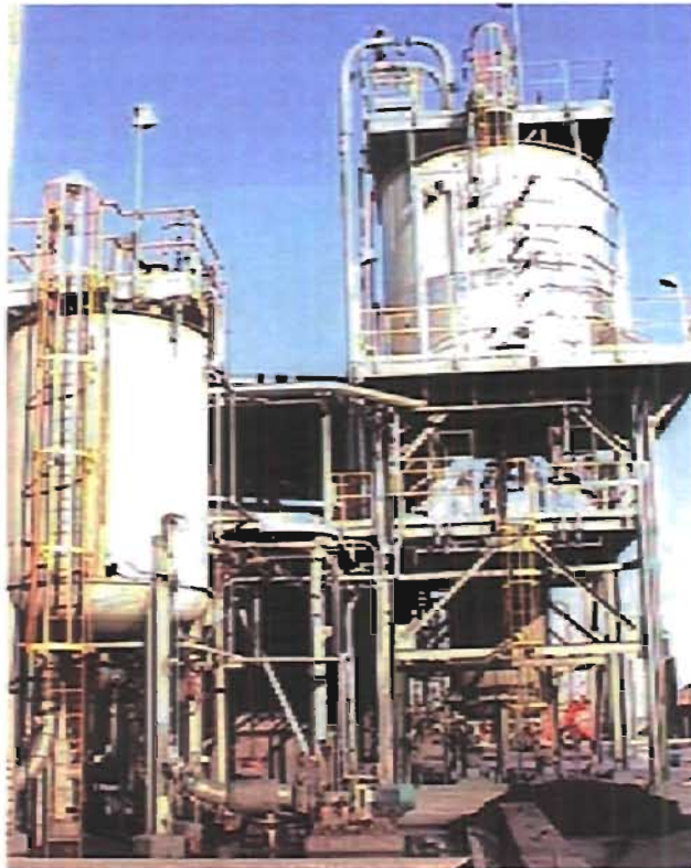
Figure 1-16 New Settler Feed Tank (Left) and Settler (Right)
