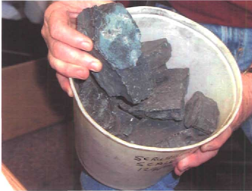
Figure 1-15 Hard 2 Inch Thick Scrubber Scale
