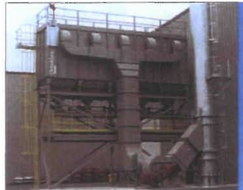
405MBT8 at a brick manufacturing facility
