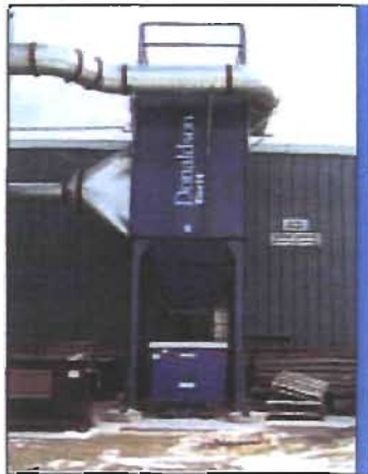
54MBTH8 at a cabinet shop on wood dust, from cutting, moulding and sanding
