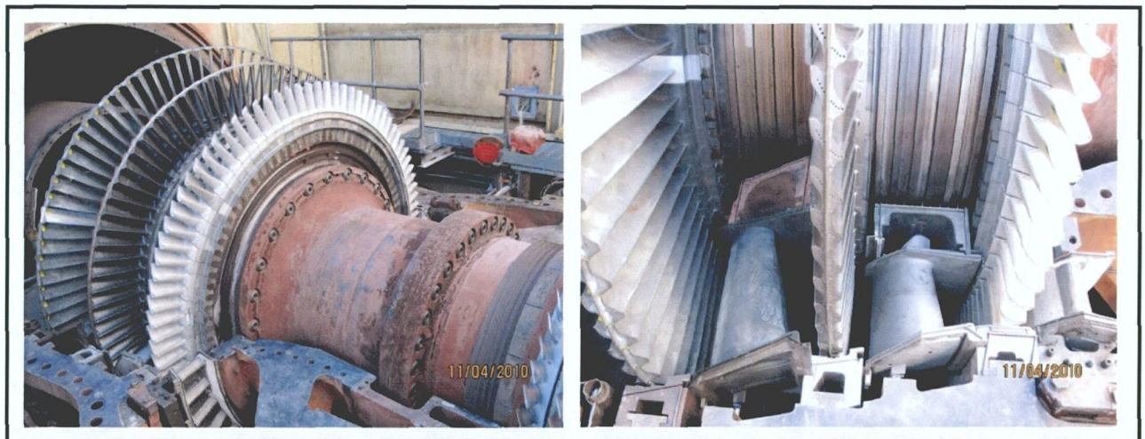
Figure 4. Internal Photo of GE 7FA with Combustors Removed. Details of Rotor Section.
