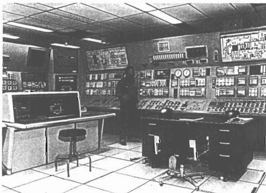
Eurocan chose Advanced Forest Automation's Autorecovery process control system for its project. The recovery boiler control panel is on the right side and the Autorecovery operator's station on the left.
