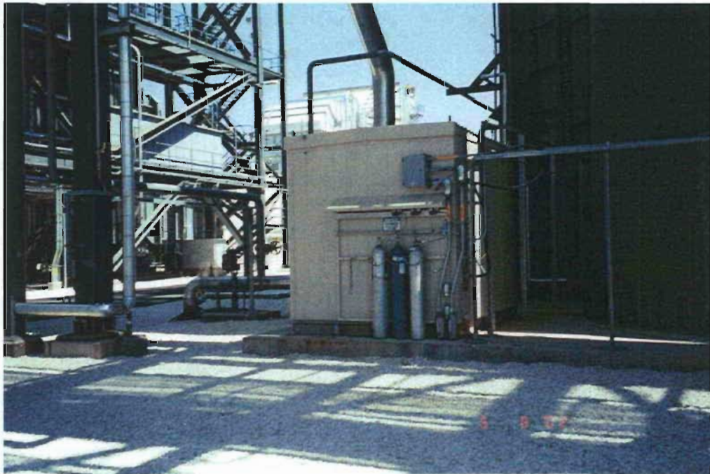
Unit 5A CEM Shelter
