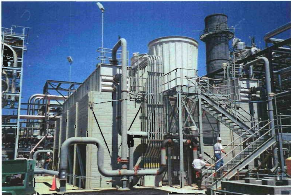
Wet Surface Air Cooler (Unit 5). Unit 5B stack in background.
