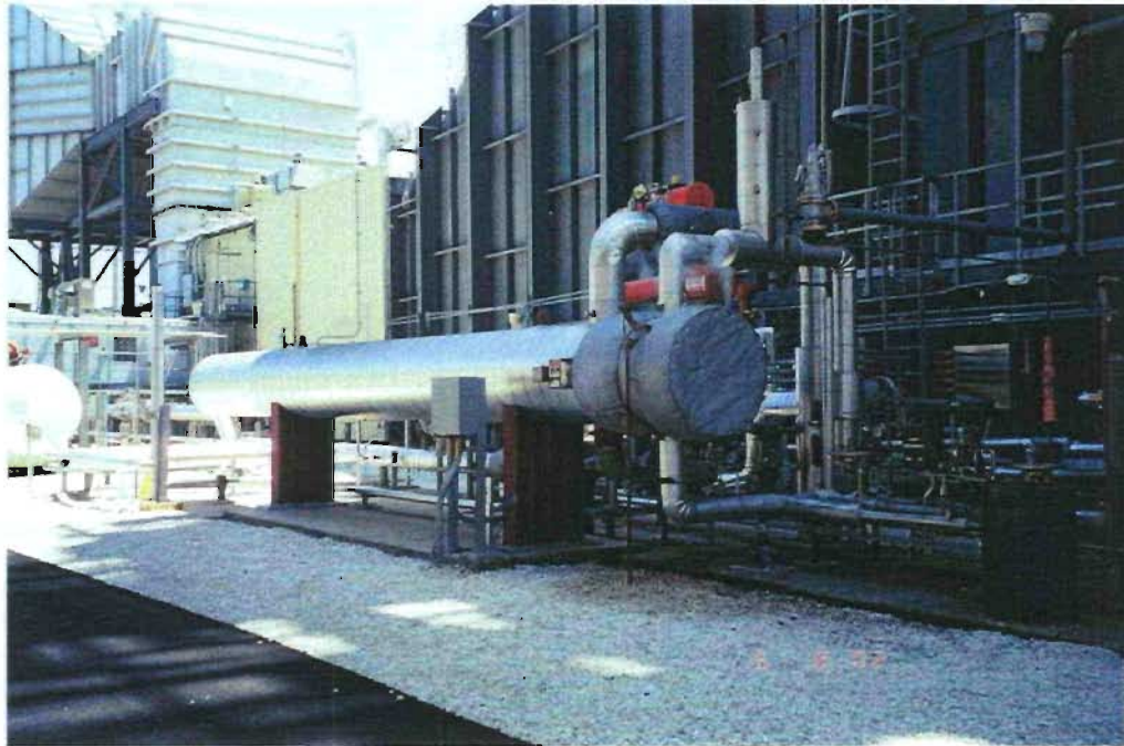
Unit 5A Steam Gas Heater
