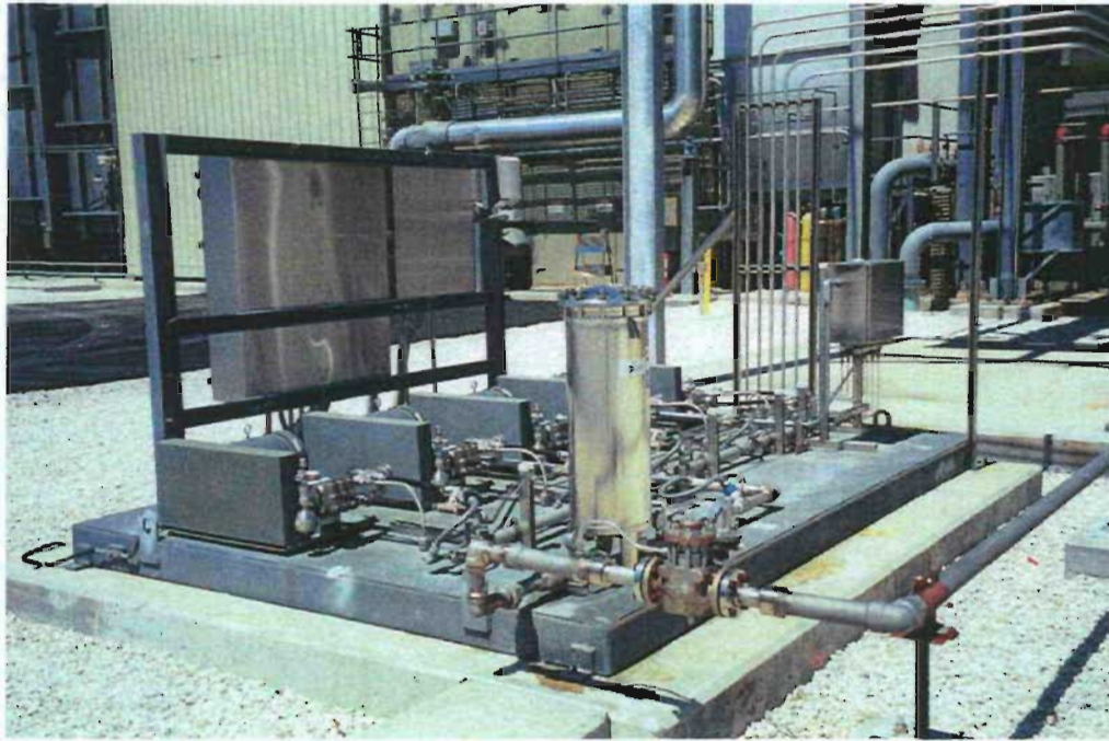
Unit 5A Inlet Fogger Skid
