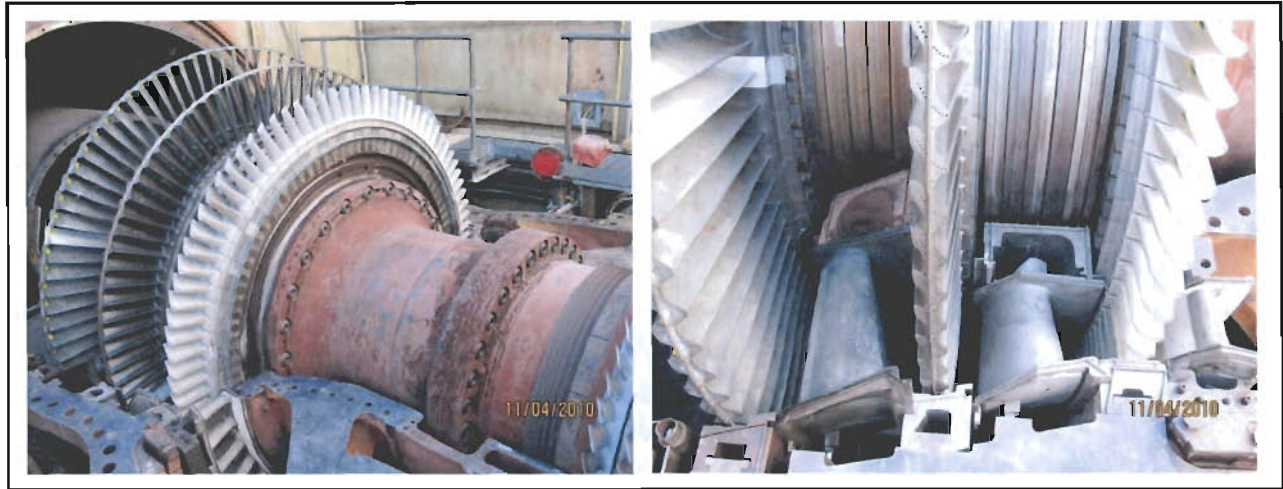
Figure 4. Internal Photo of GE 7FA with Combustors Removed. Details of Rotor Section.
