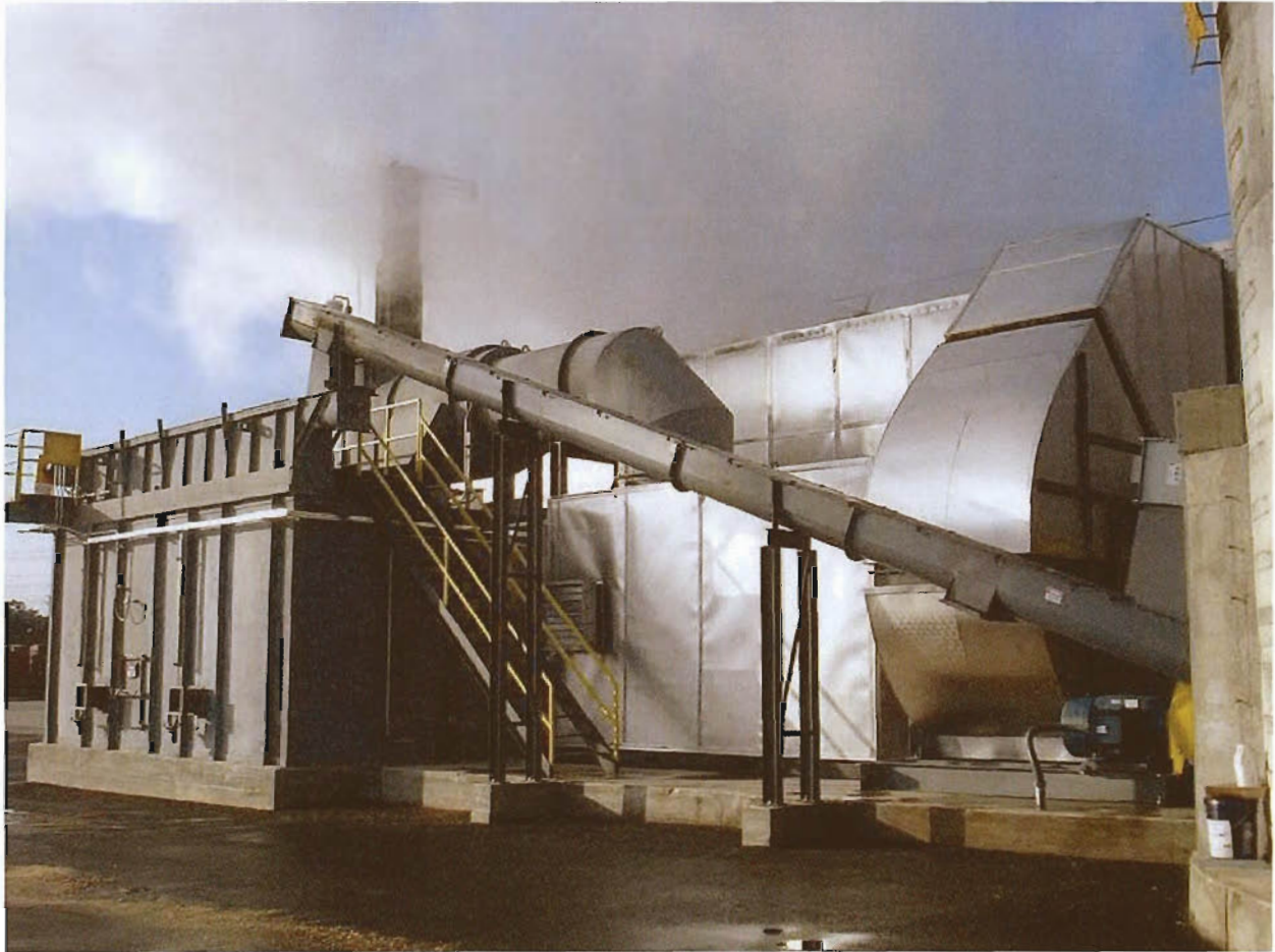
KDS RECIRCULATION AIR SYSTEM, MIXING CHAMBER AND BURNER SYSTEM
