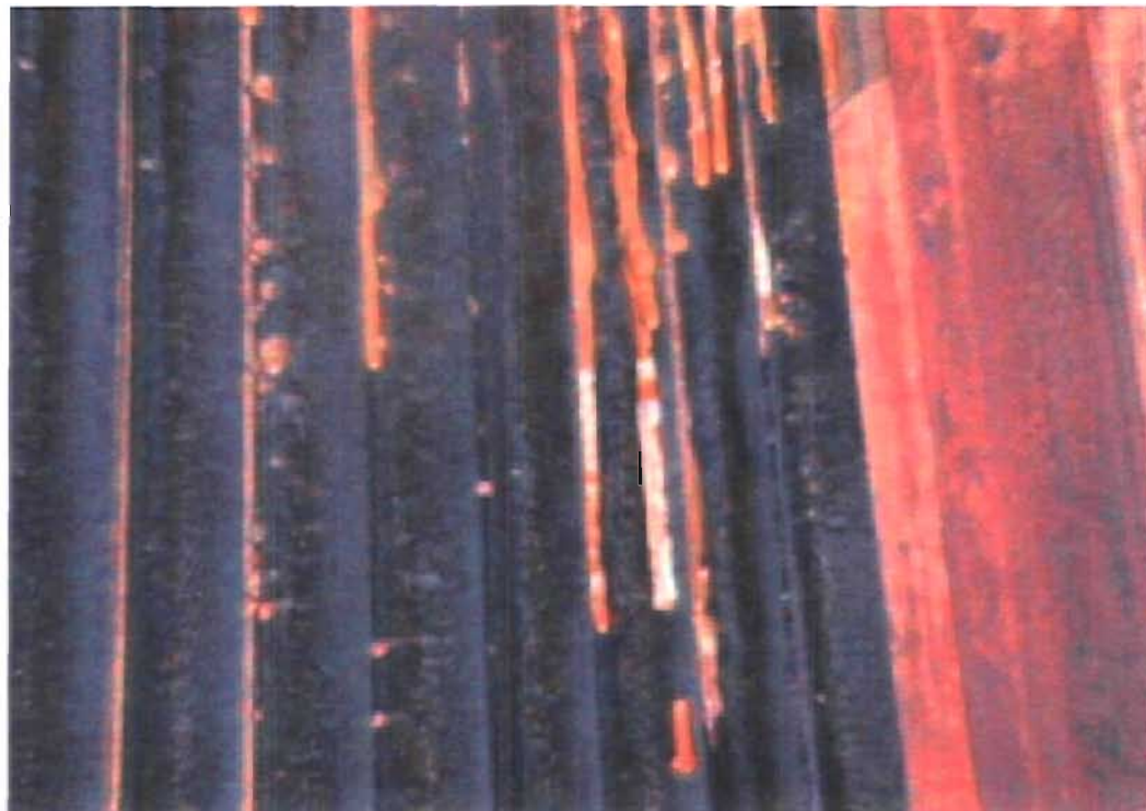
Deposits in the HRSG, low-pressure section of economizer
