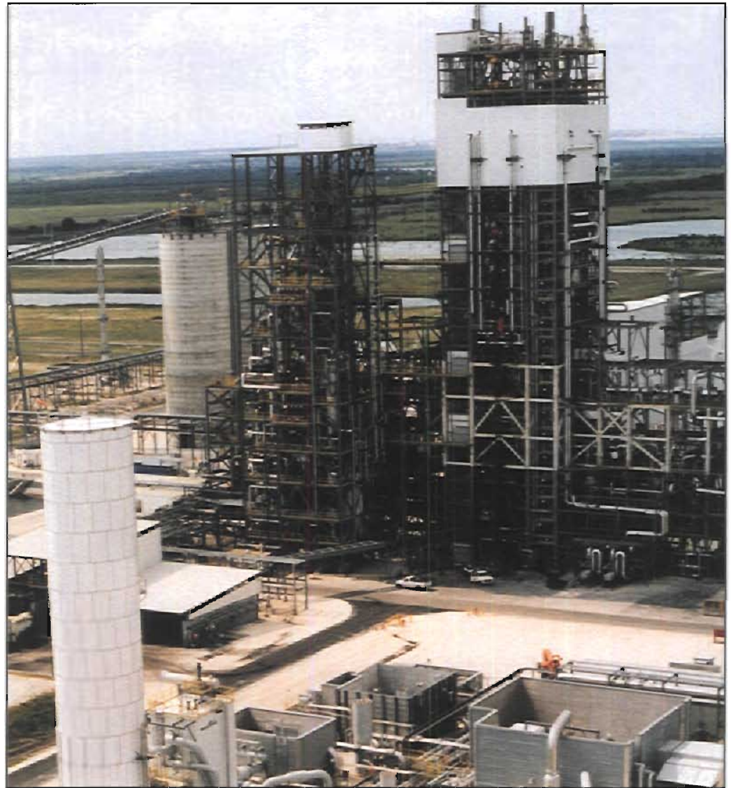
The Texaco gasifier is in the largest structure, which also contains the radiant syngas cooler. The hot gas cleanup system is installed in the smaller of the two large structures. In the foreground is the air separation unit.
