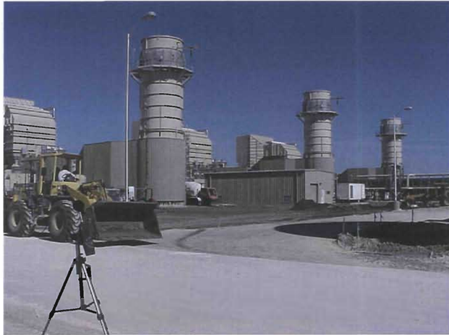
Photo 1. Diagonal View - Combustion Turbine
