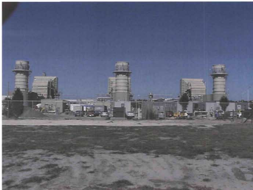
Photo 2. Front View - Combustion Turbine
