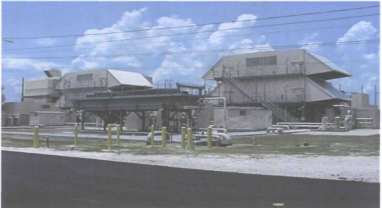
Photo 1. Combustion Turbine Units 7 and 9
