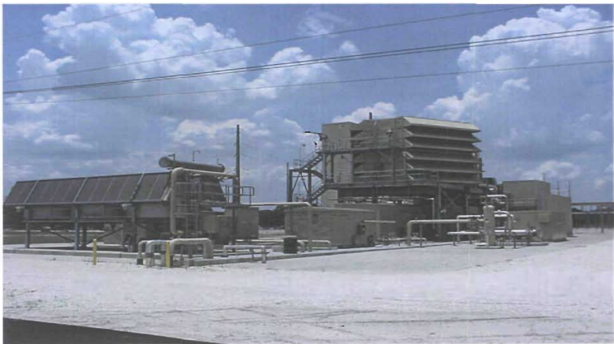
Photo 2. Combustion Turbine Peaking Unit 13
