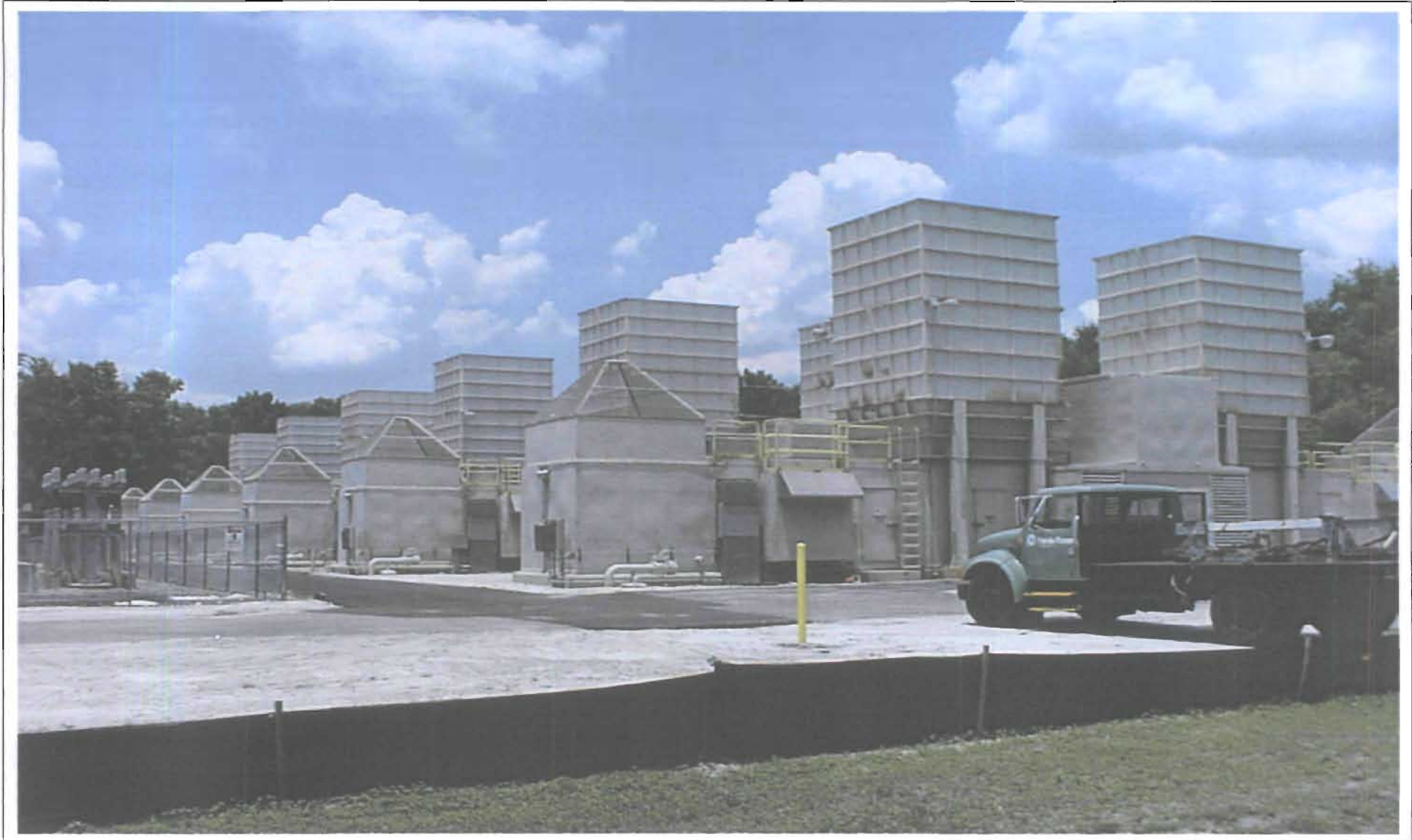
Attachment IC-EU1-A9 Combustion Turbine Peaking Units 1-6 Florida Power, Intercession City
