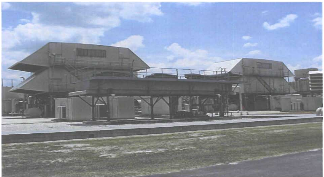
Photo 2. Combustion Turbine Units 8 and 10
