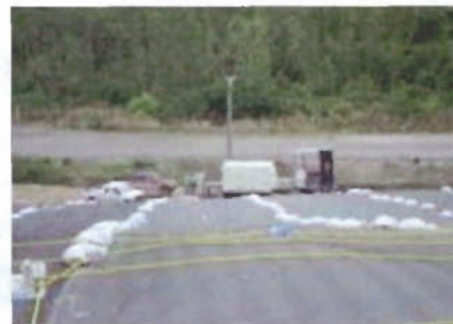
Figure 6 – Relocatable Odor Flare
