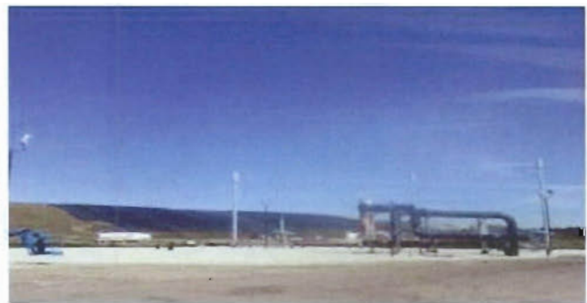
Figure 9 – Piping to Planned GDP, New Open Flares
