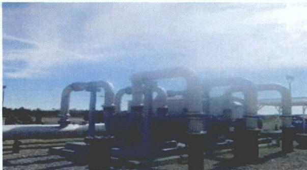
Figure 8 – Conditioned LFG Piping
