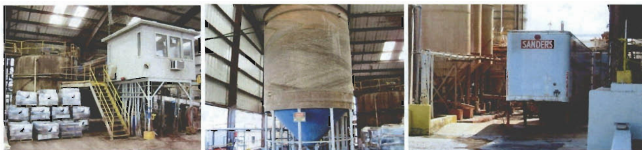
Figure 7. Settling tank & control room, sulfuric acid storage, trailer awaiting load of plastics.
