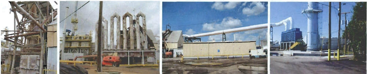
Figure 11. Afterburner; cooling loops, baghouses, stacks; negative air baghouse with stack.
