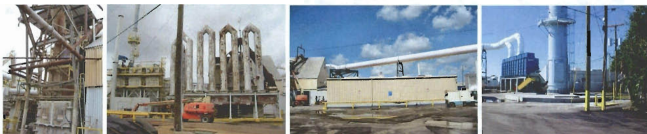
Figure 11. Afterburner; cooling loops, baghouses, stacks; negative air baghouse with stack.
