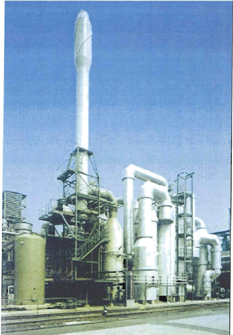
Tail gas cleaning unit based on the Peracidox ® process for a 330 mtpd Mh double-catalysis plant based on spent acid decomposition.
