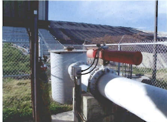
Figure 4 - Flare Knock-Out Drum Main Inlet Valve
