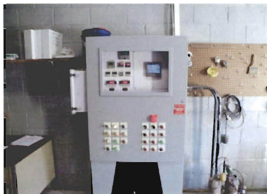
Figure 7 - Flare Control Panel
