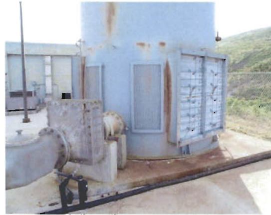
Figure 6 - Flare Flame Arrestor & Louvers
