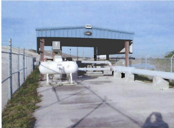
Figure 3 - Flare Propane Tank
