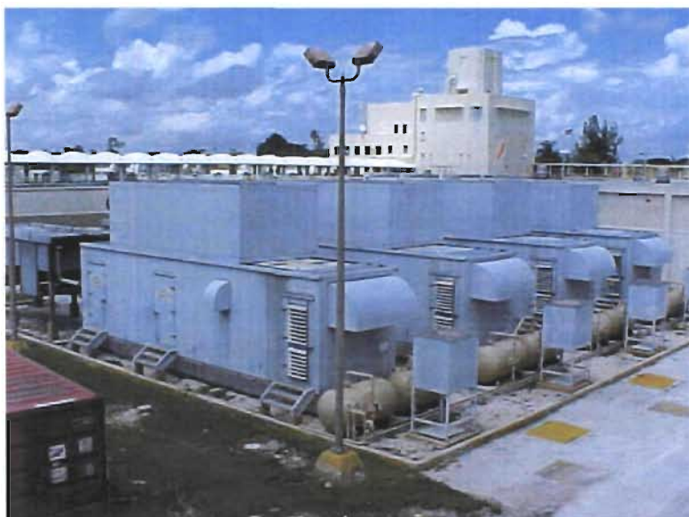
Figure 3-2 Alexander Orr, Jr. WTP Standby Generator Bank
