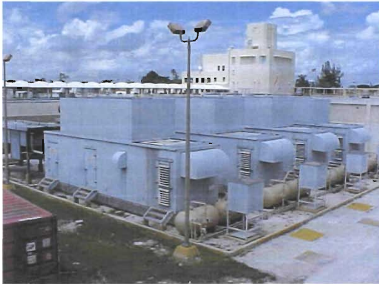
Figure 3-2 Alexander Orr, Jr. WTP Standby Generator Bank
