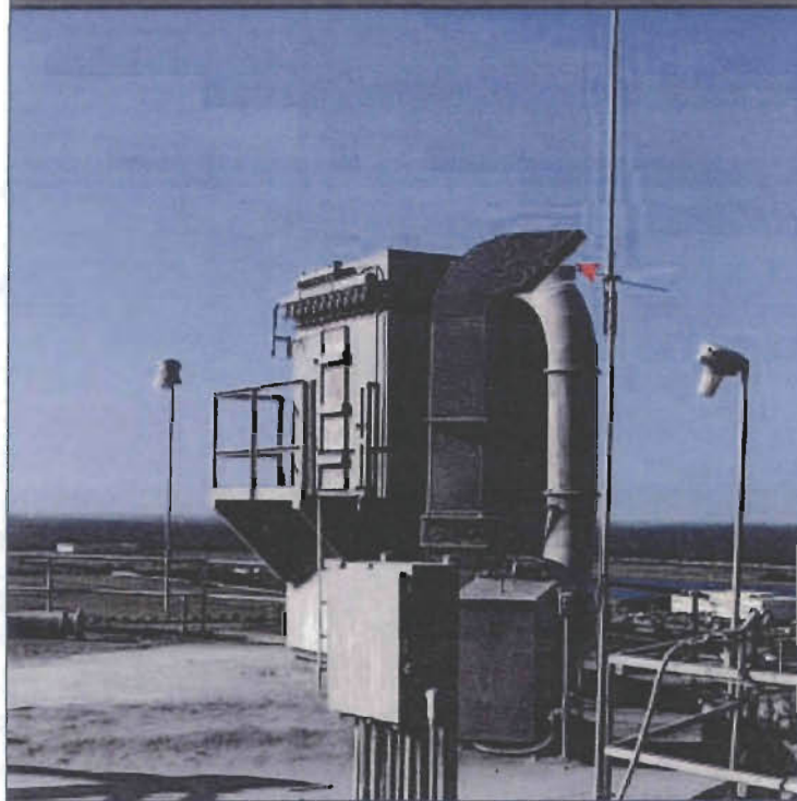
Emission Control Equipment Aug05
