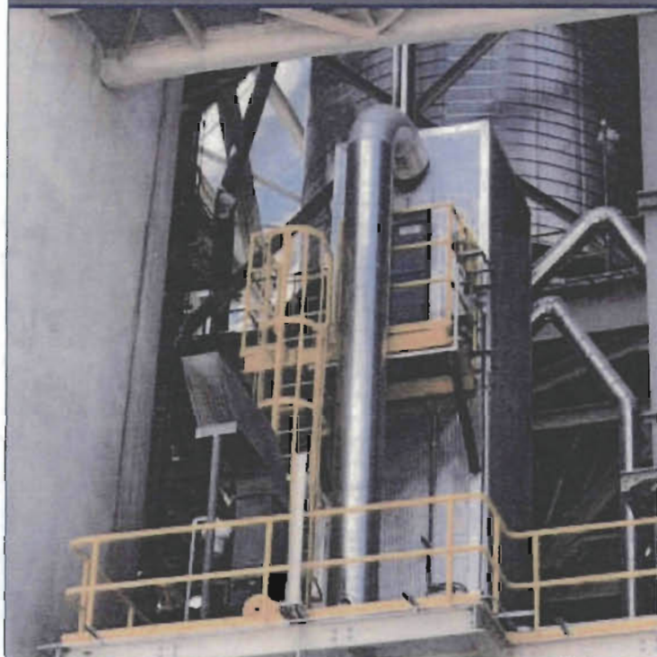
Emission Control Equipment Aug05
