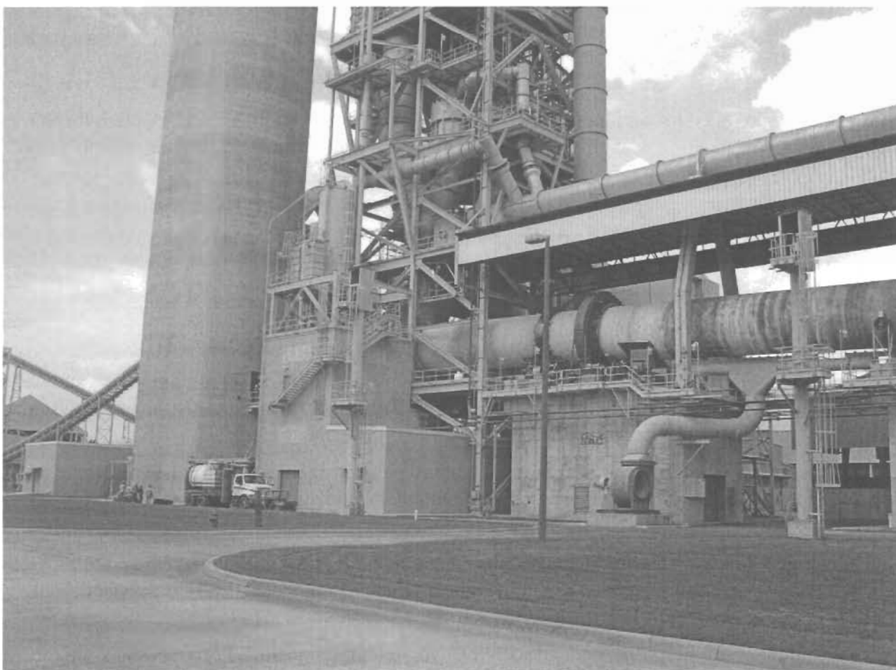
Kiln Inlet, Main Stack, Lower Preheater, Calcliner, and Tertiary Air Ducts (Photo A. Linero)
