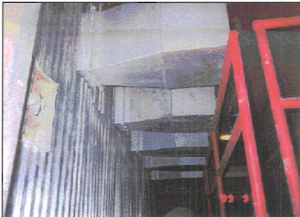
Photo 1. OFA Nozzles on the East Wall
