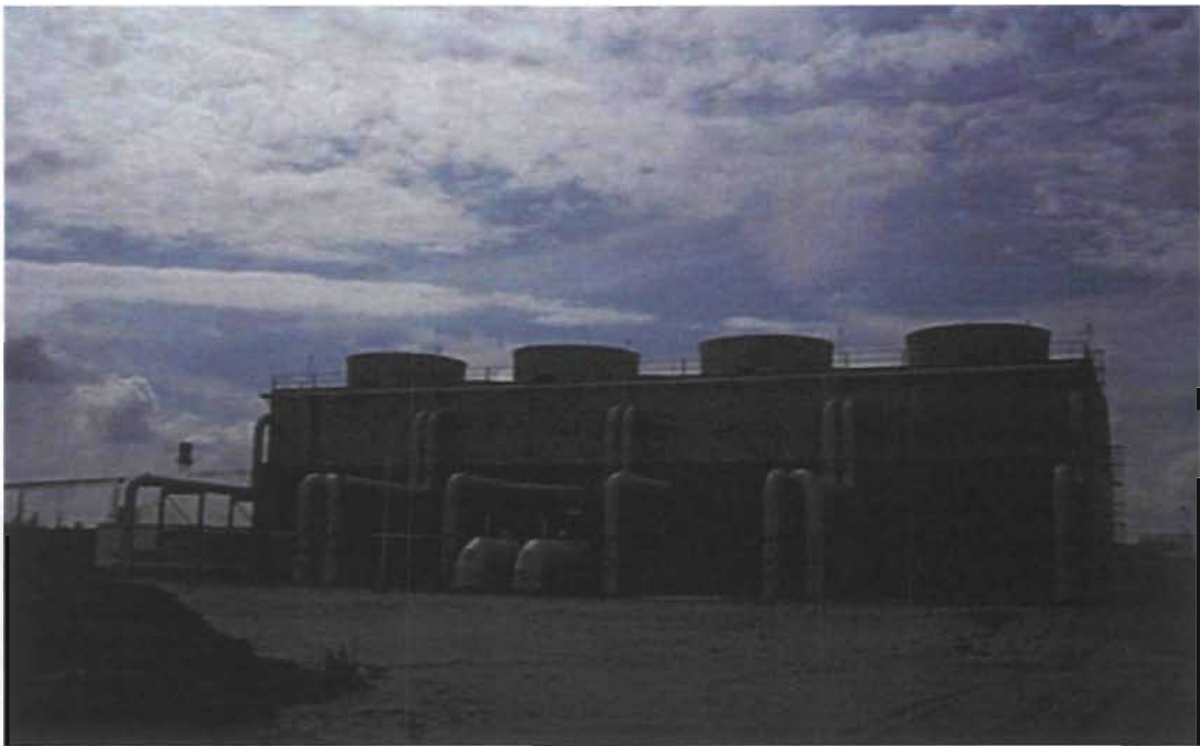
Photo 2. Close View - Cooling Towers
