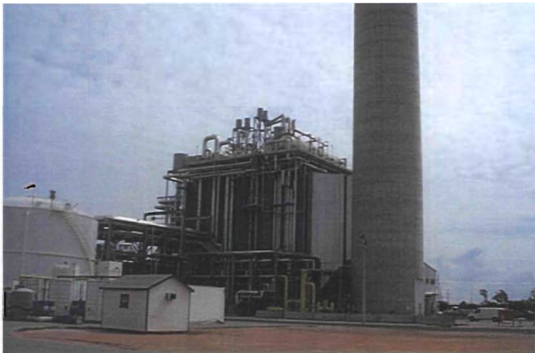
Photo 2. Unit 5 HRSG and Stack – View Toward Northeast
