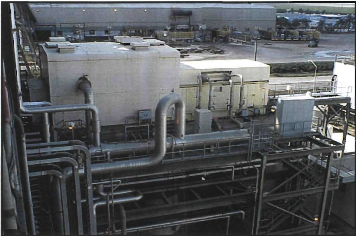
Figure 3.2-3d. NHPP Existing Steam Turbine/Electric Generator.
