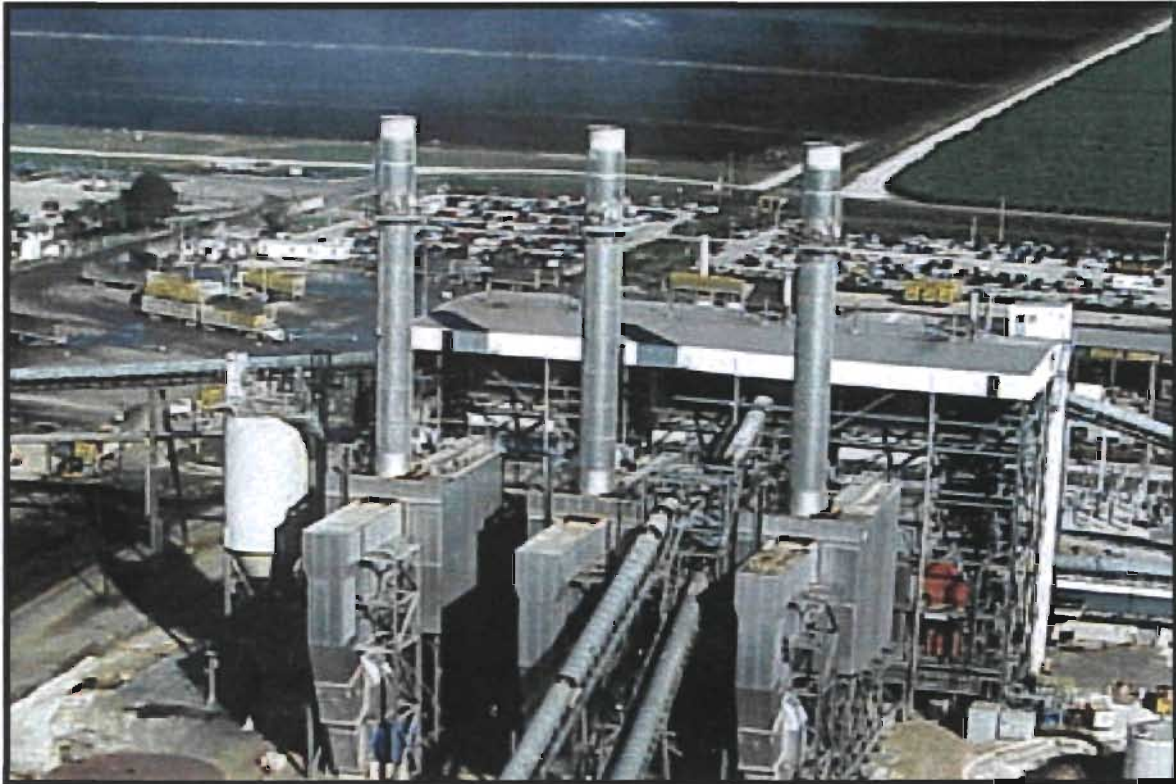
3.2-3c. NHPP Existing Biomass Boilers (view looking north).
