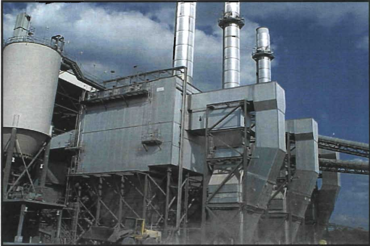
Figure 3.2-3e. NHPP Boilers Electrostatic Precipitators (ESPs).
