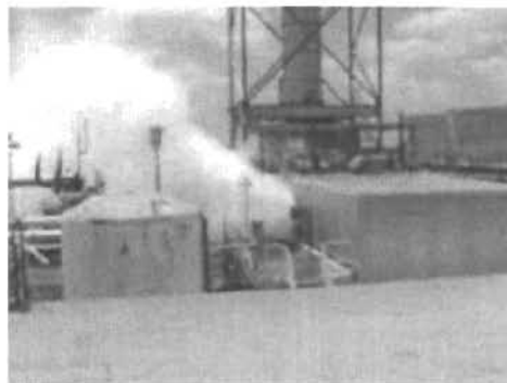
Figure 2. Malfunction event, steam leaking from Unit S-3.
