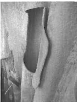
Figure 1. Leak in external water-wall.
