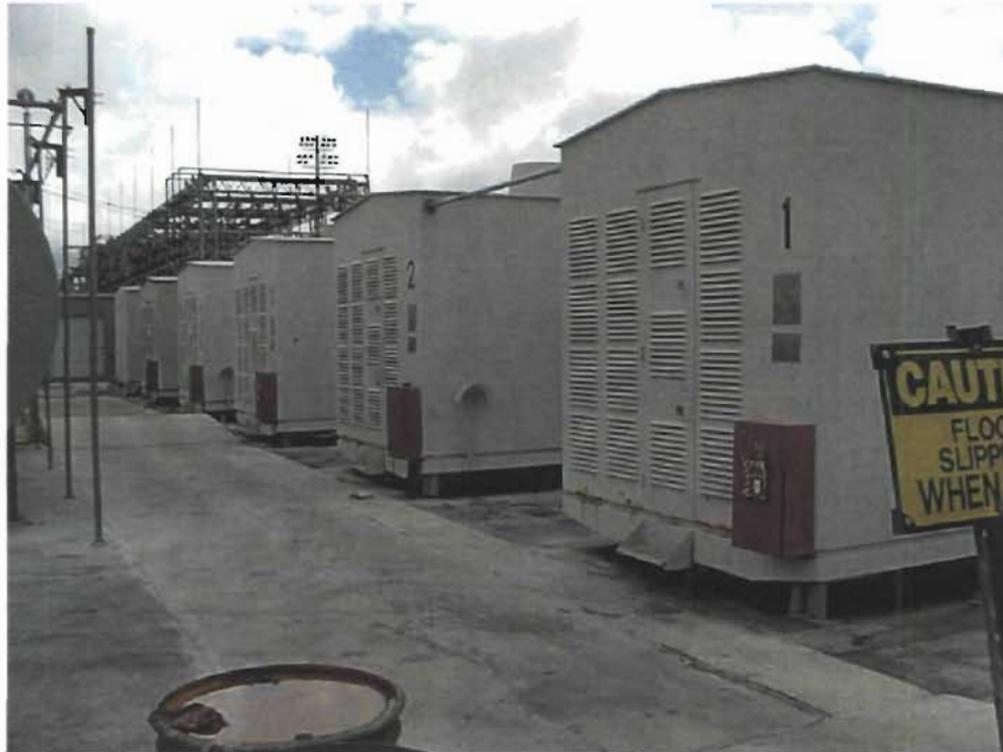
Photo 1. Front View - Diesel Generator Units 1-5
