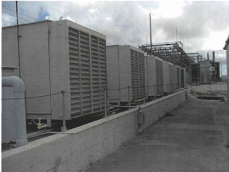
Photo 2. Rear View - Diesel Generator Units 1-5
