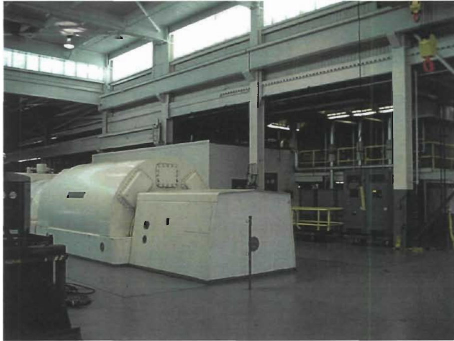
Photo 1. Inside View - Turbine and Generator for Unit S-3
