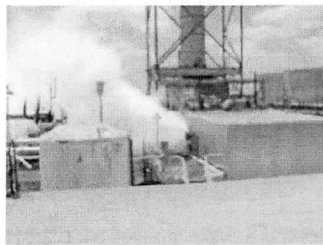
Figure 2. Malfunction event, steam leaking from Unit S-3.
