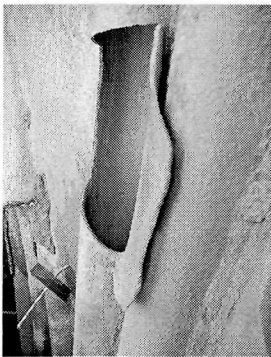
Figure 1. Leak in external water-wall.
