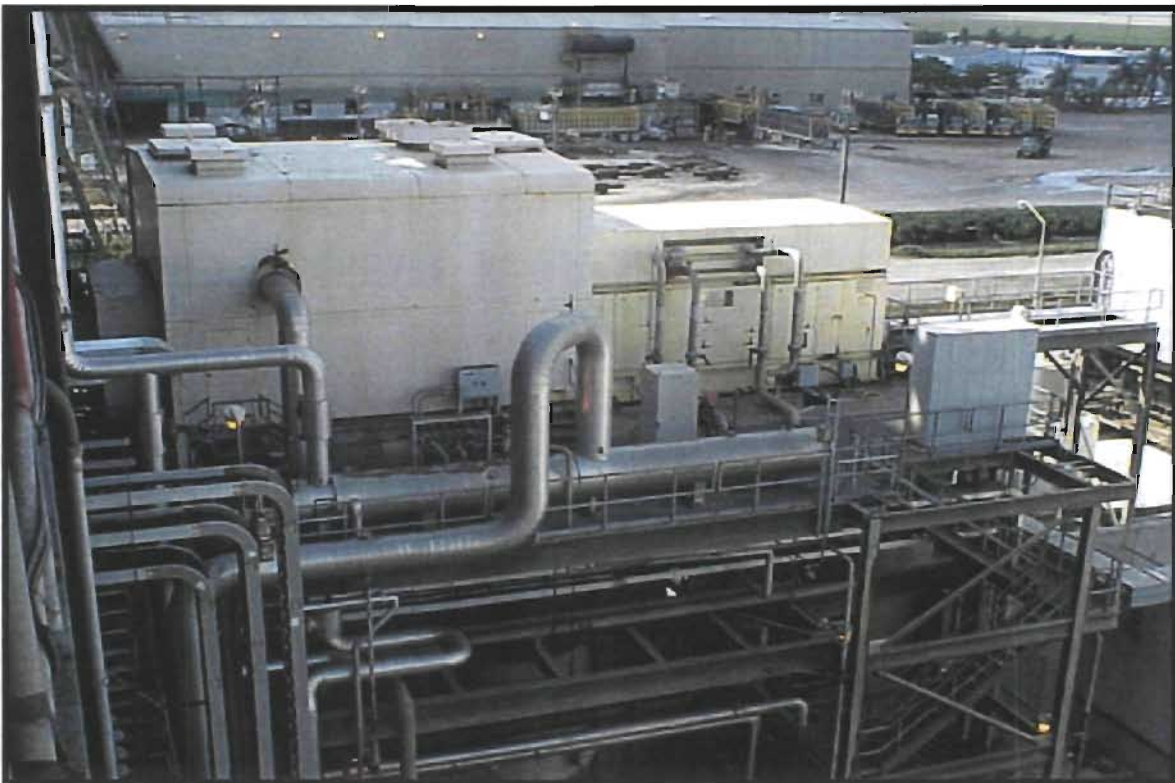
Figure 3.2-3d. NHPP Existing Steam Turbine/Electric Generator.
