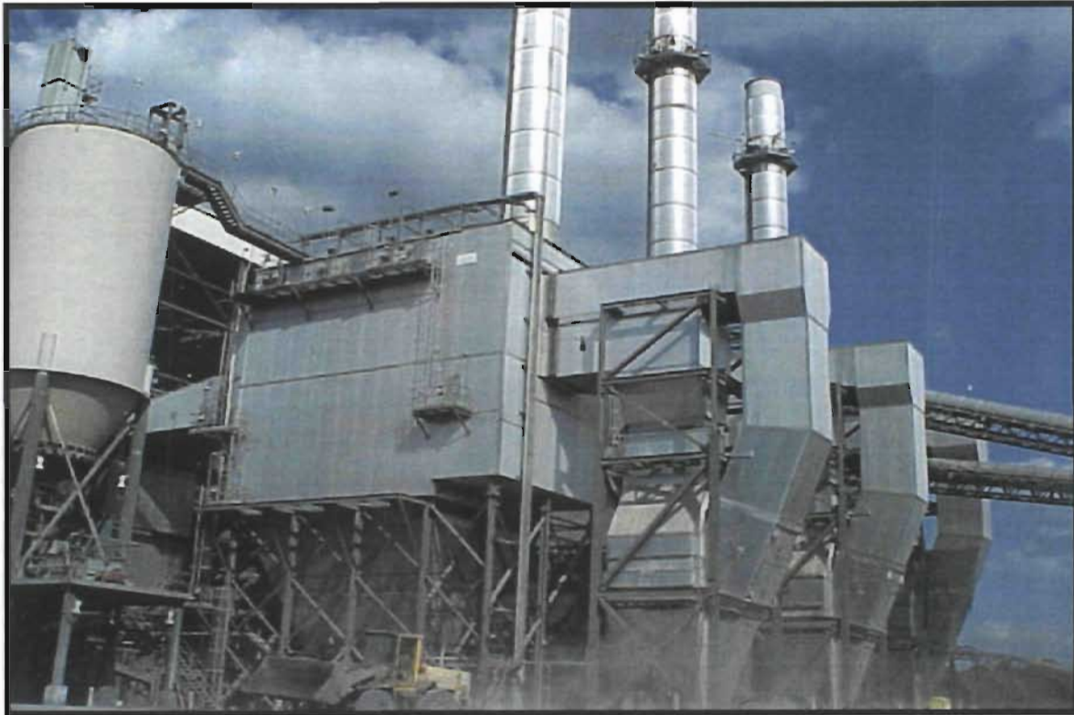
Figure 3.2-3e. NHPP Boilers Electrostatic Precipitators (ESPs).
