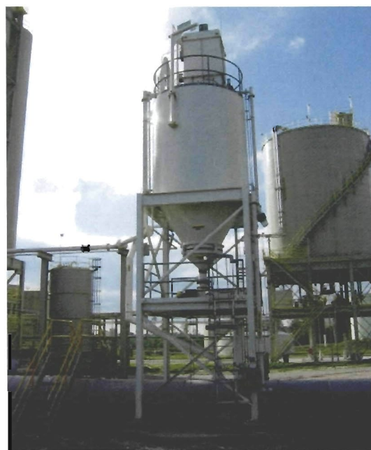
Figure 3 - Sorbent Injection System at GRU.
