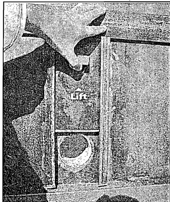
Access Hole (DO NOT TOUCH DOOR IF IT IS HOT)
