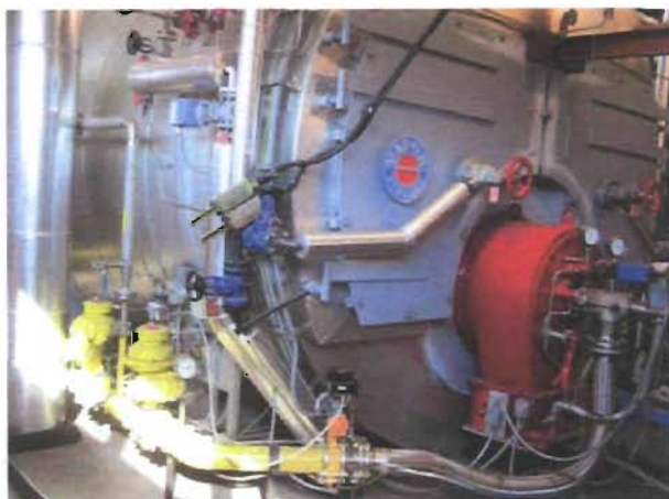
Figure 8: Oulun Energia's 5MW Boiler at Oulu University Hospital where LFG is used to provide process steam for sterilization purposes. Oulun Energia produces electricity and heat.
