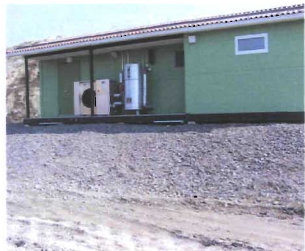
Figure 5: Water chiller unit, utilizing refrigeration principles, used for drying the gas. The picture shows the housing for the pumping plant on the new-landfill site. The plant has a capacity of 500Nm 3 /h.
