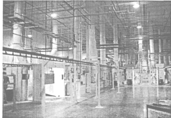
Hanging Chain Finishing Conveyor Line
