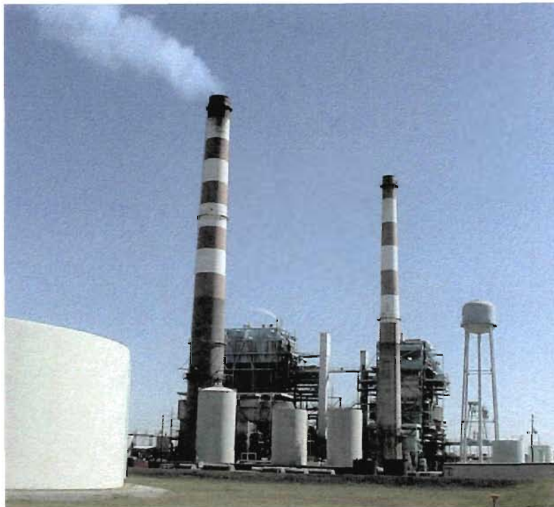
Figure 3 – Existing Residual Oil Fired Units to be Replaced
