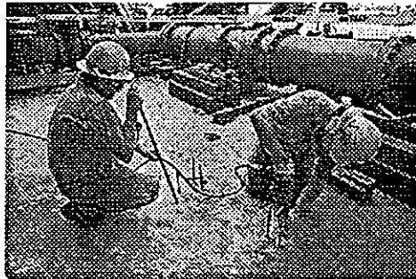
Roy Goss, left, and Scott Subbert prepare foundations to mount heat exchangers at the Florida Power & Light plant in Fort Myers last week. Subbert is a mechanic for mechanical maintenance at the plant and Goss is maintenance leader. Lisa Krantz/Staff
