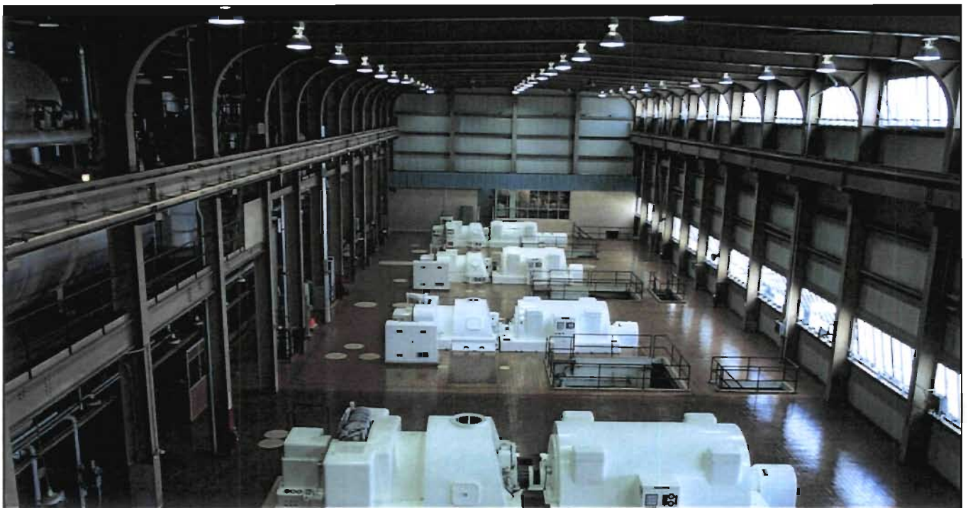
Photo 4. Steam Generator Units 1 - 4
