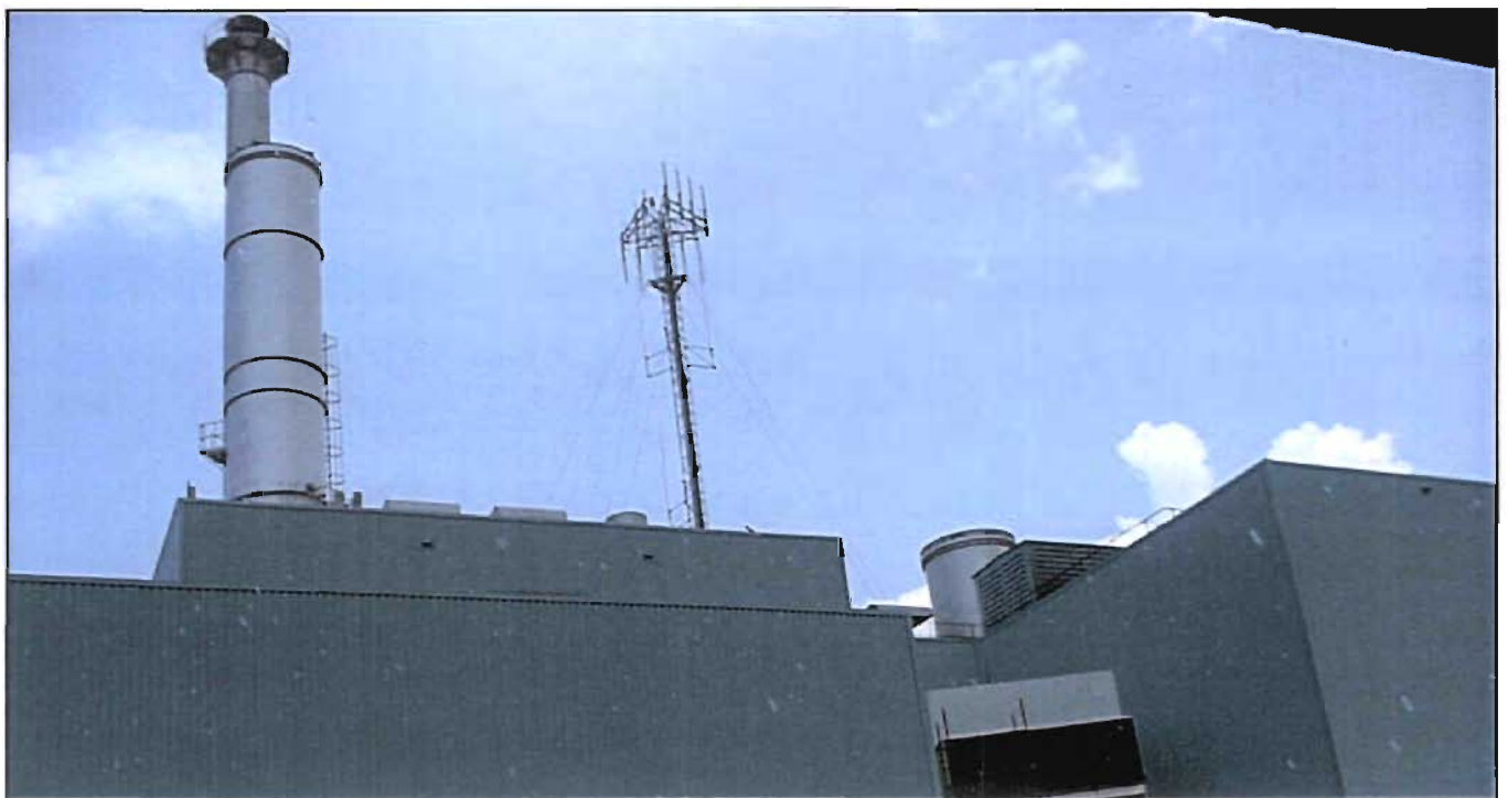
Photo 6. Simple Cycle and Combined Cycle Stacks for Unit 5
