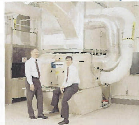
Ray Gryniewicz, Technical Equipment Manager, Facilities, of Chrysler Corporation and Todd Ainsworth, Sales Engineer of Tri-Mer Corporation with one of the eight systems installed at Chrysler Tech Center.
