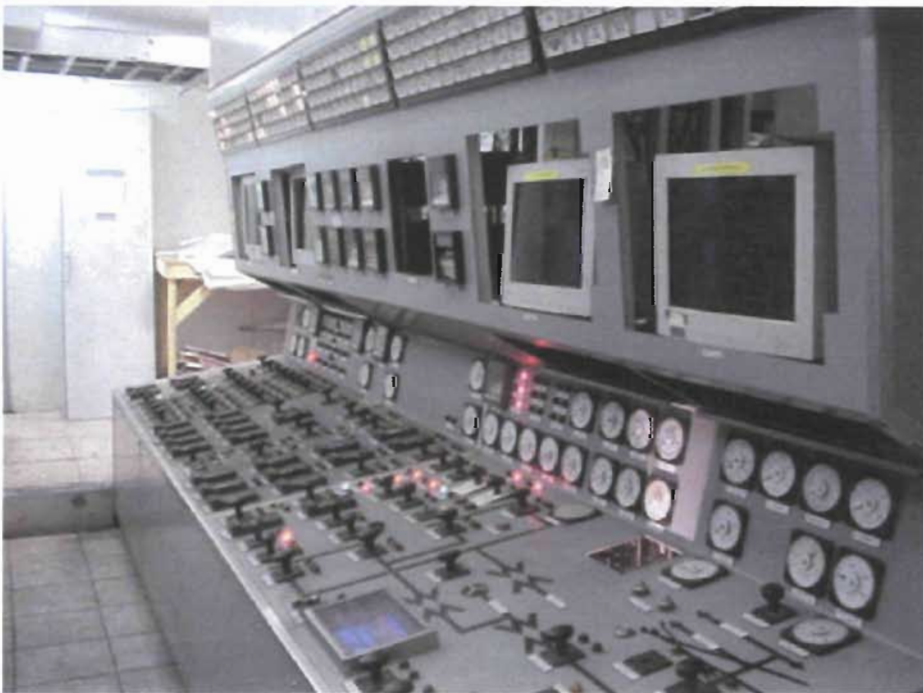
Picture #4. TECO-Gannon Plant control room
