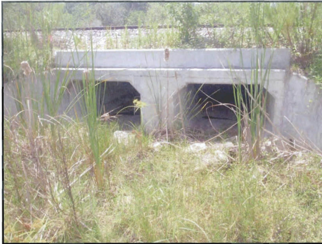
Photograph No. 17. View of culverted railroad crossing which drains Wetland W1 looking west from edge of Wetland W1.
