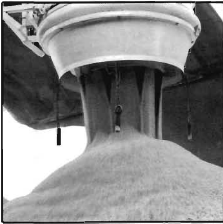
Loading of potash at rates up to 1800tph at the Texas City, Texas plant of International Minerals Corp is facilitated by this MIDWEST International Chokefeeder dust control system. The Texas City terminal loads out potash, soda ash, green coke, and calcined coke and the Chokefeeder enables the facility to comply with standards set by the Environmental Protection Agency of the United States without covering the hatch.
