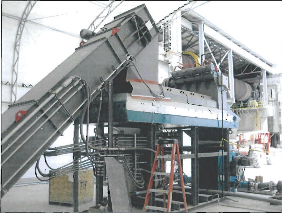
FIGURE 6. CONVEYORS COMING FROM OFFLOADING PORTS TO METERING SYSTEM.
