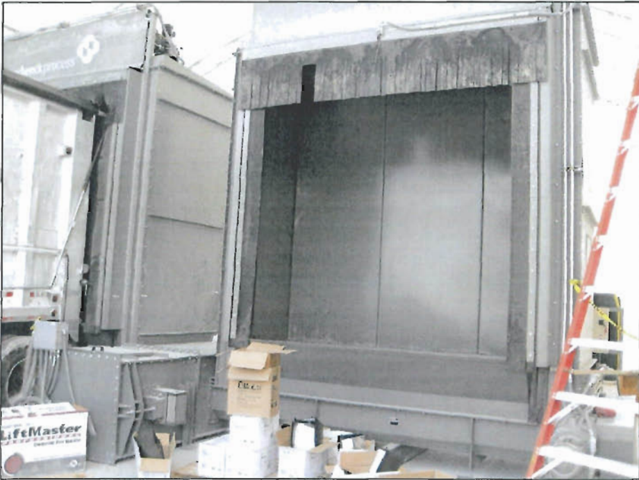
FIGURE 4. TWO OFFLOADING PORTS OF TYPICAL SCHENK FEEDER SYSTEM
