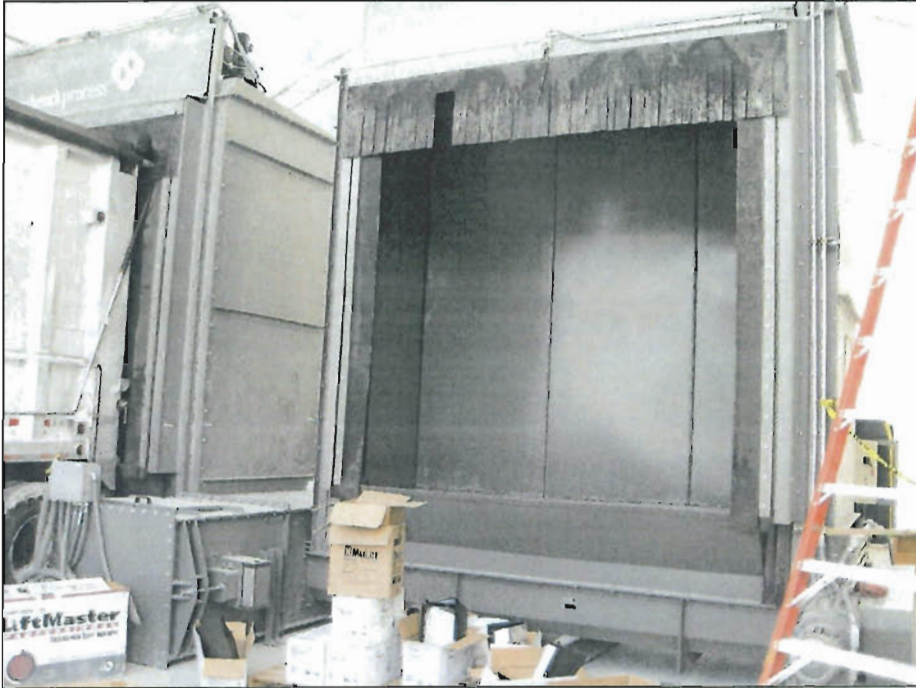
FIGURE 4. TWO OFFLOADING PORTS OF THE SCHENCK FEEDER SYSTEM
