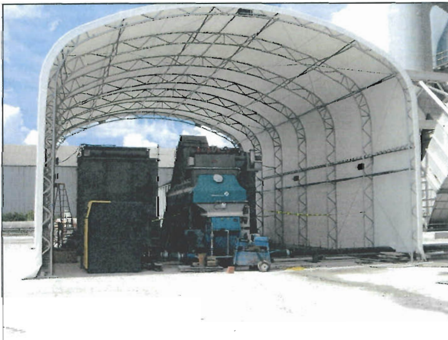
FIGURE 3. SCHENK FEEDER SYSTEM OF THE BIOMASS AT THE MIAMI CEMENT PLANT
