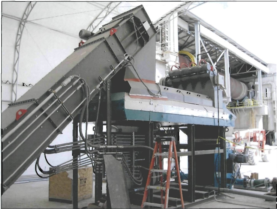
FIGURE 4. CONVEYORS COMING FROM OFFLOADING PORTS TO METERING SYSTEM.
