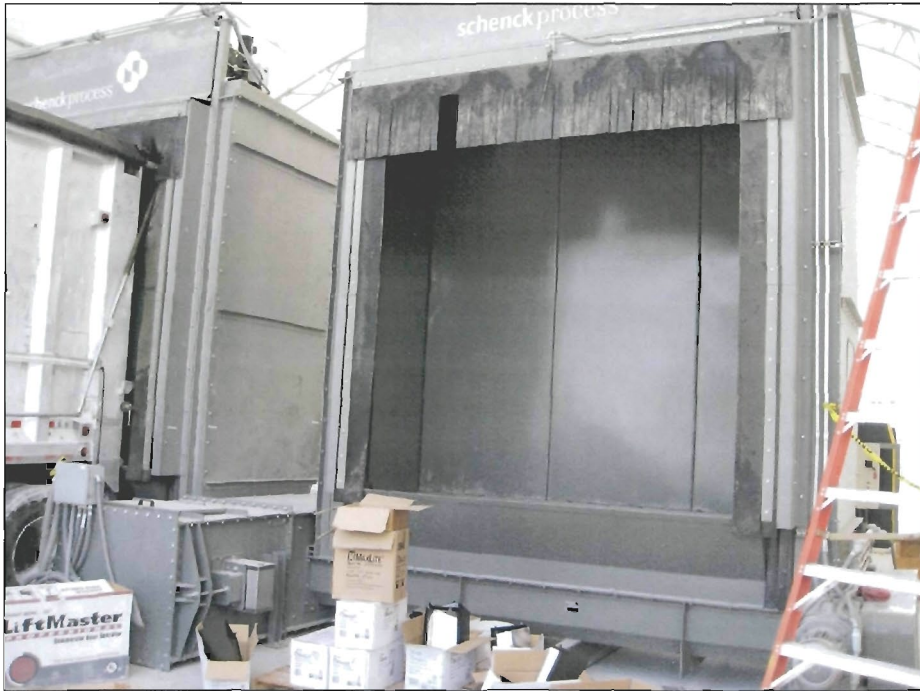
FIGURE 2. TWO OFFLOADING PORTS OF THE SCHENCK FEEDER SYSTEM
