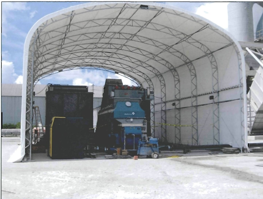
FIGURE 1. SCHENK FEEDER SYSTEM OF THE BIOMASS AT THE MIAMI CEMENT PLANT
