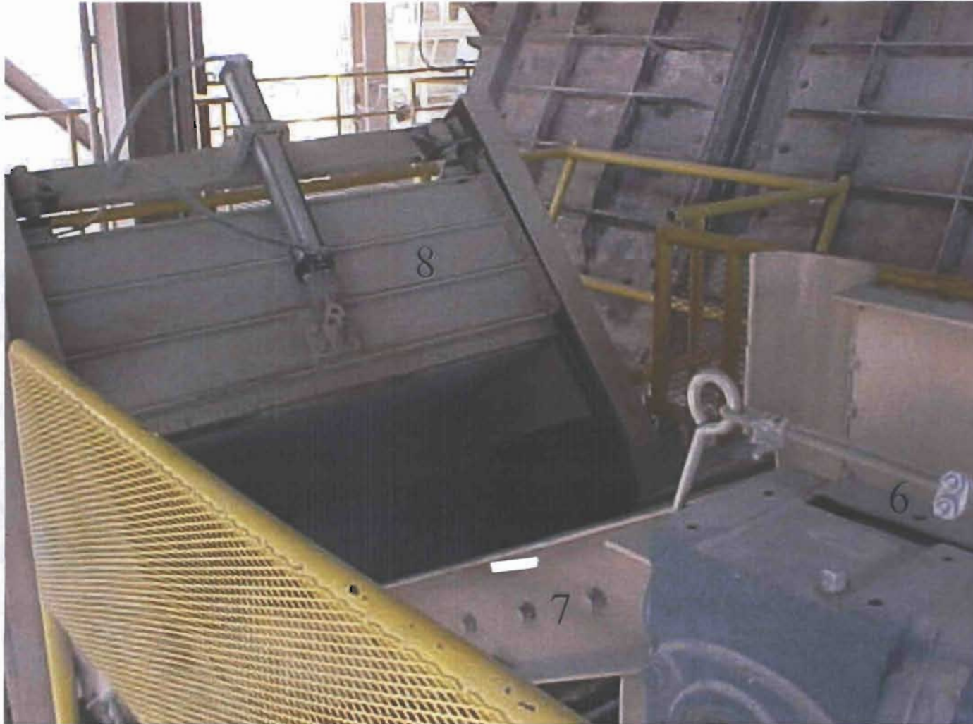
6 - Cross-Belt Conveyor 7 - Scale 8 - Double Gate
