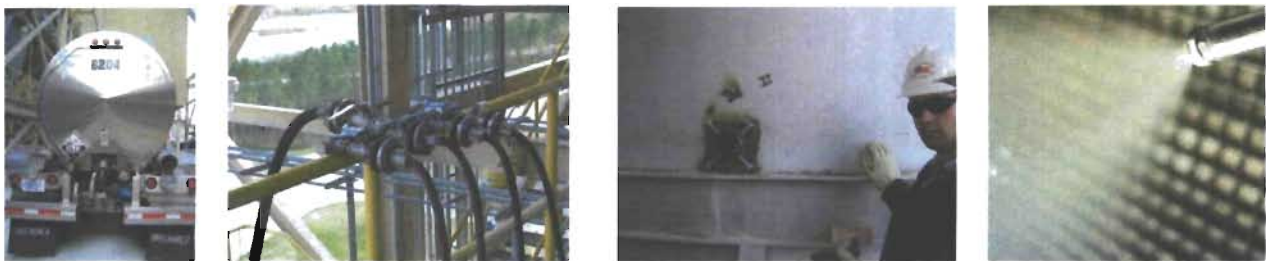
Figure 7. Aqueous Ammonia Supply Truck, Compressed Air, One of Four Ports, an Injector
