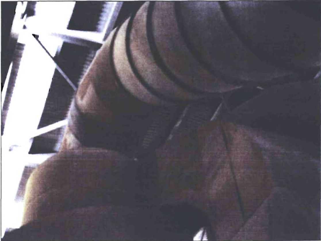
Figure 20: Raw Mill #2 by pass Ducting (1).
