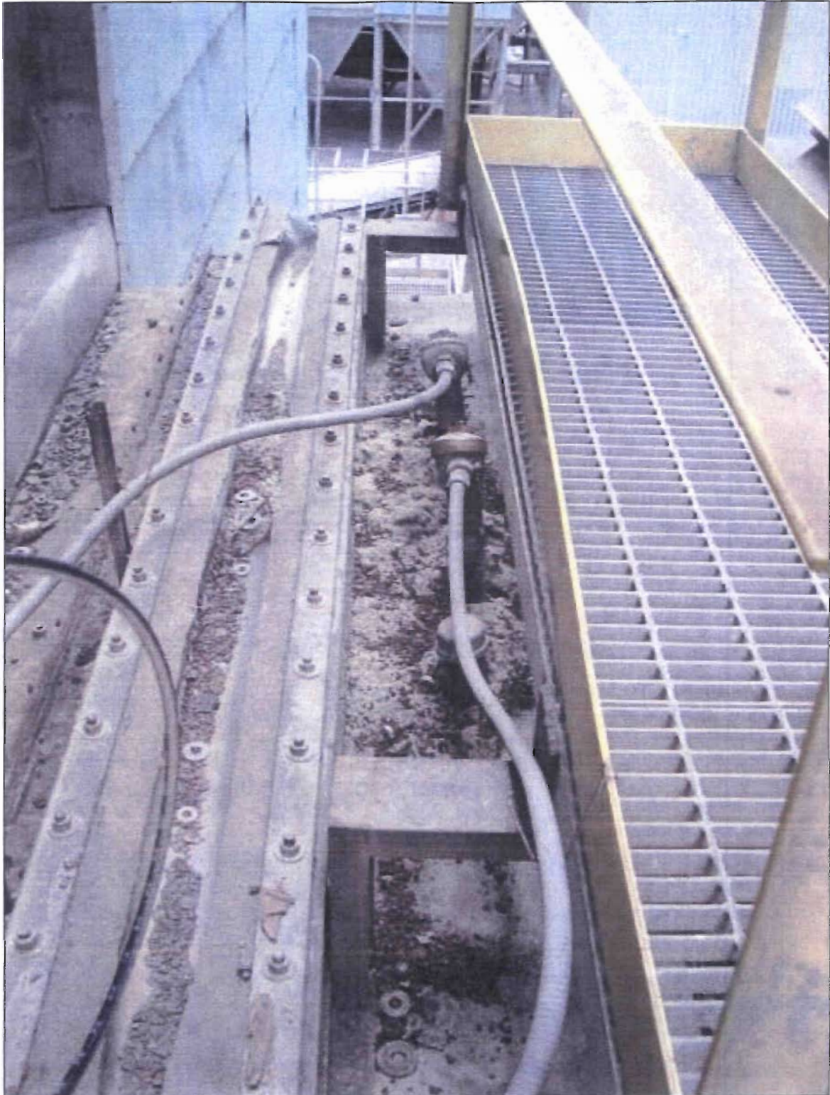
Figure 12: #2 Kiln—Raw Mill BH Inlet Thermocouples.
