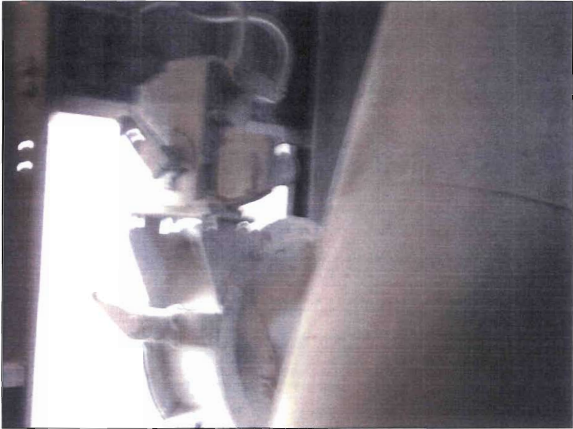
Figure 17: Raw Mill #2 2322 Damper.
