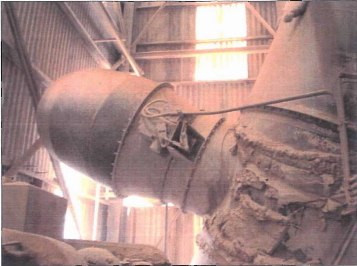
Figure 5: Old not used Raw Mill #1 323 Damper.
