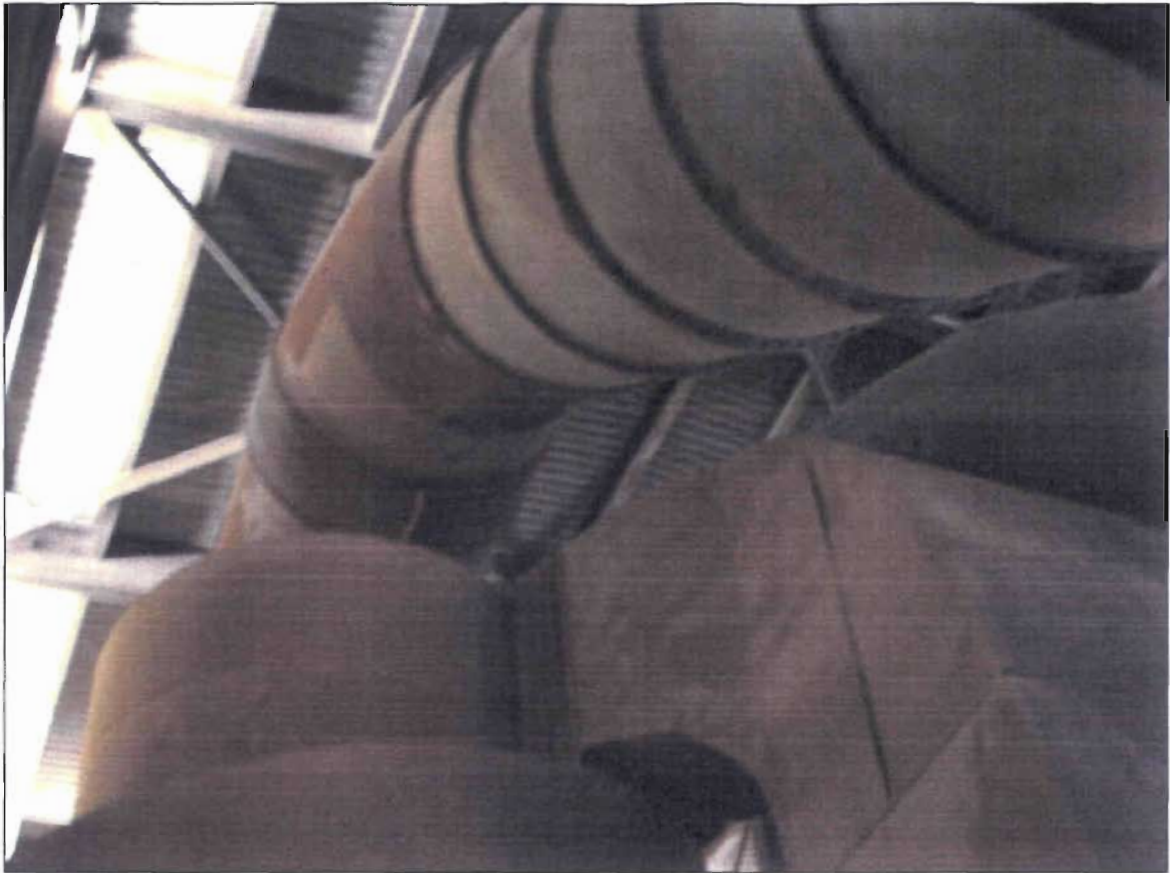
Figure 20: Raw Mill #2 by pass Ducting (1).
