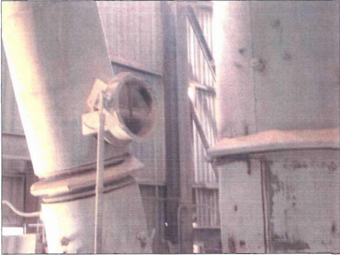
Figure 11: Raw Mill #1 322 Damper.
