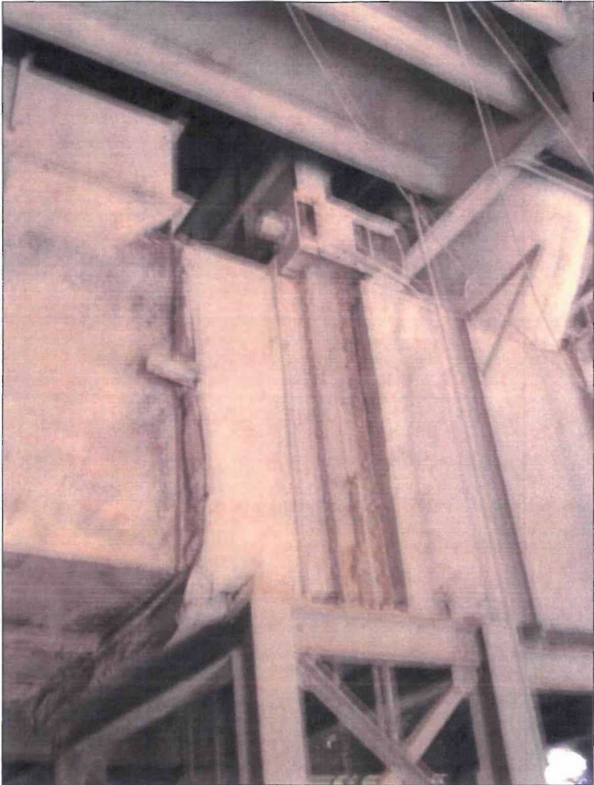
Figure 15: Raw Mill #2 2320 Damper.
