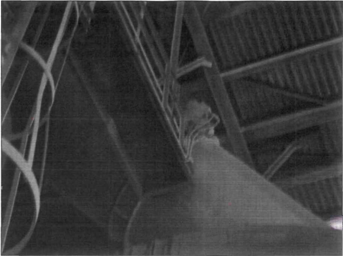
Figure 16: Raw Mill #2 2321 Damper.
