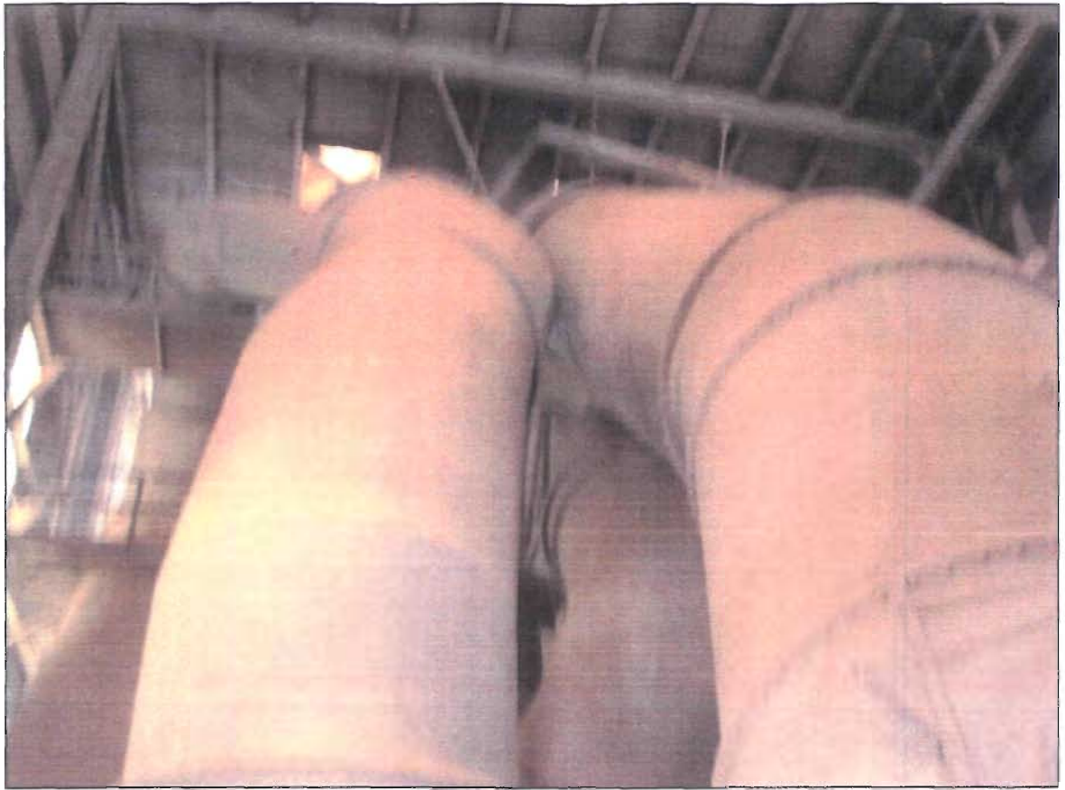
Figure 2: #1 Raw Mill by pass Ducting (1).
