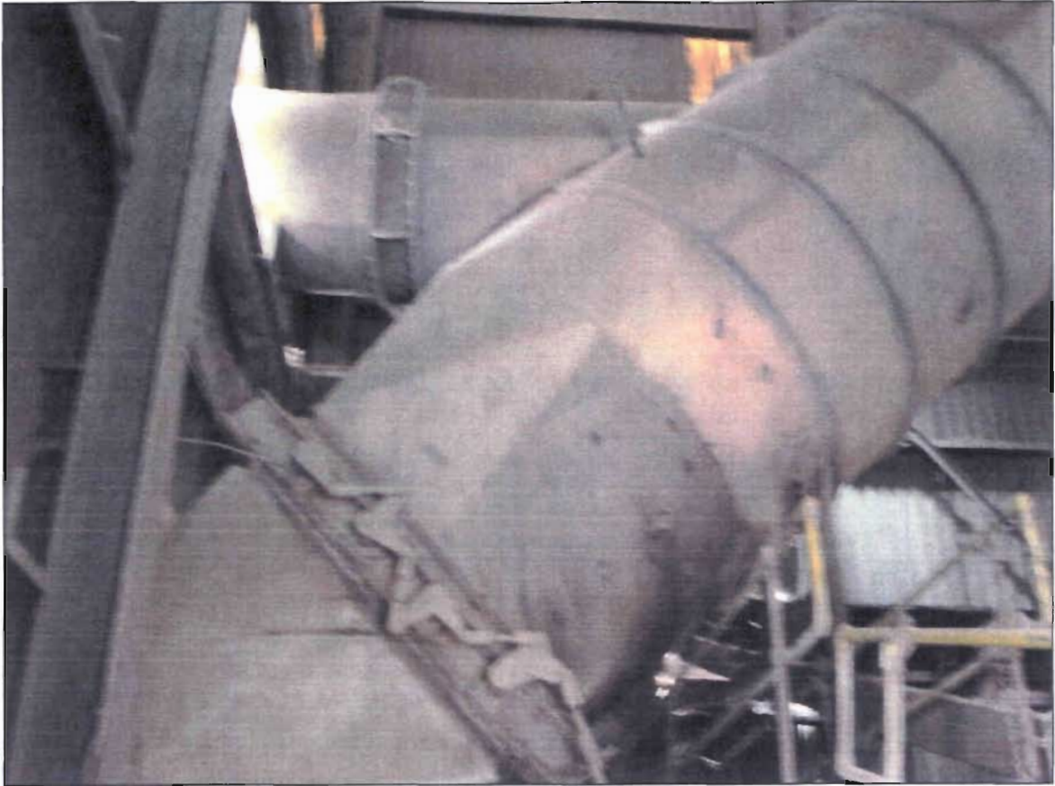
Figure 18: Raw Mill #2 2323 Damper top, 2319 Damper bottom.
